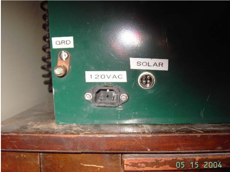
A close up showing the ground, AC, and Solar power connections.
